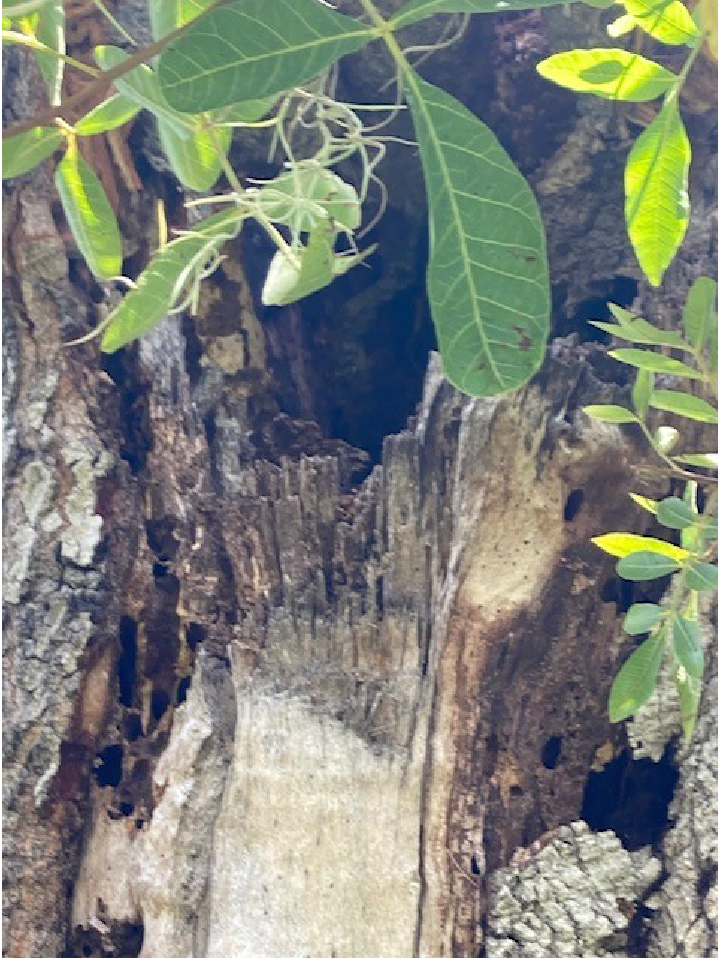
Specimen to the right of 3620 Woodmont Drive is hollow in the middle making whole tree failure more likely
