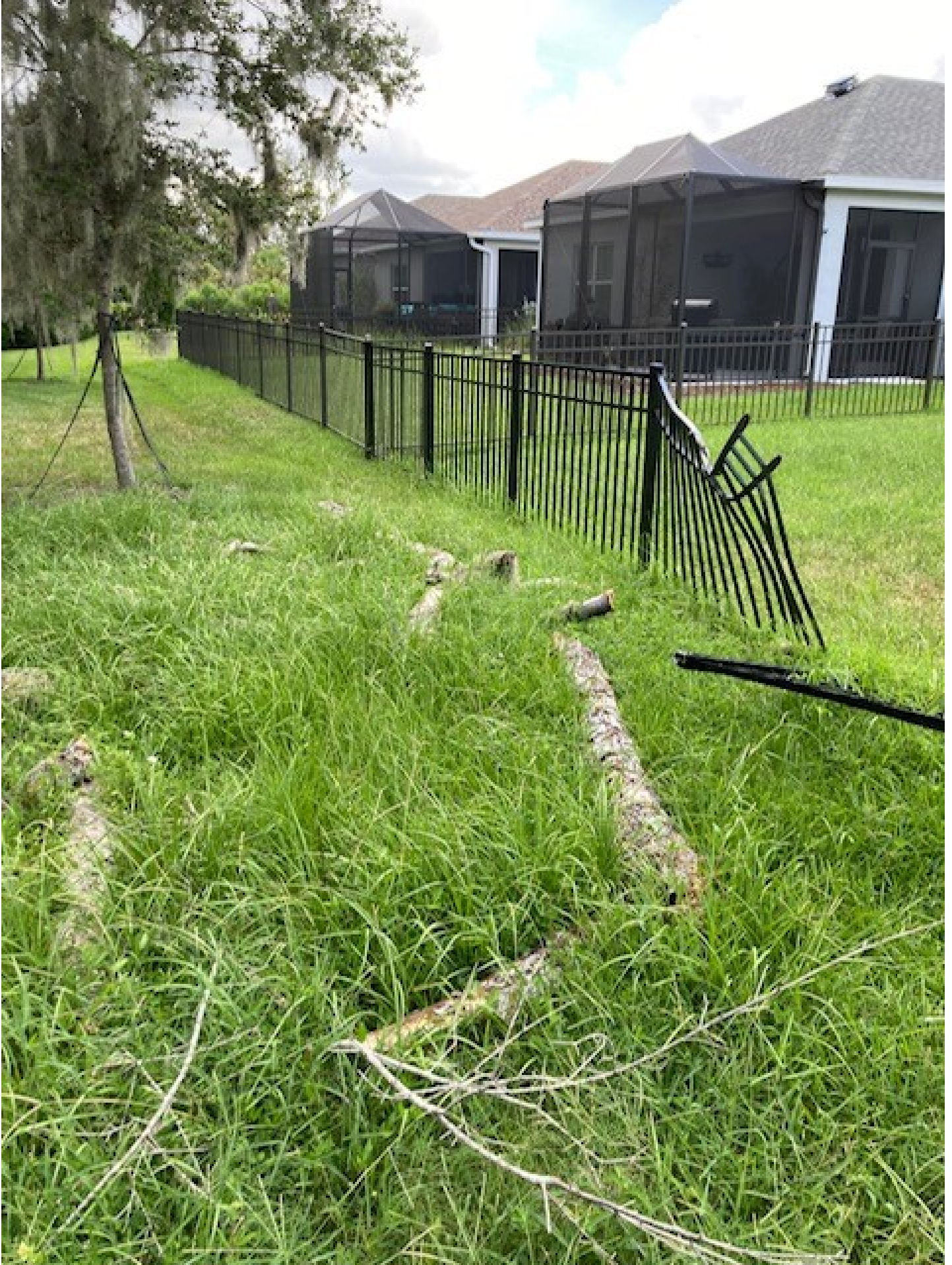
Additional Fractures in area of Fence damage from Dead Oak behind 4840 Deep Creek
