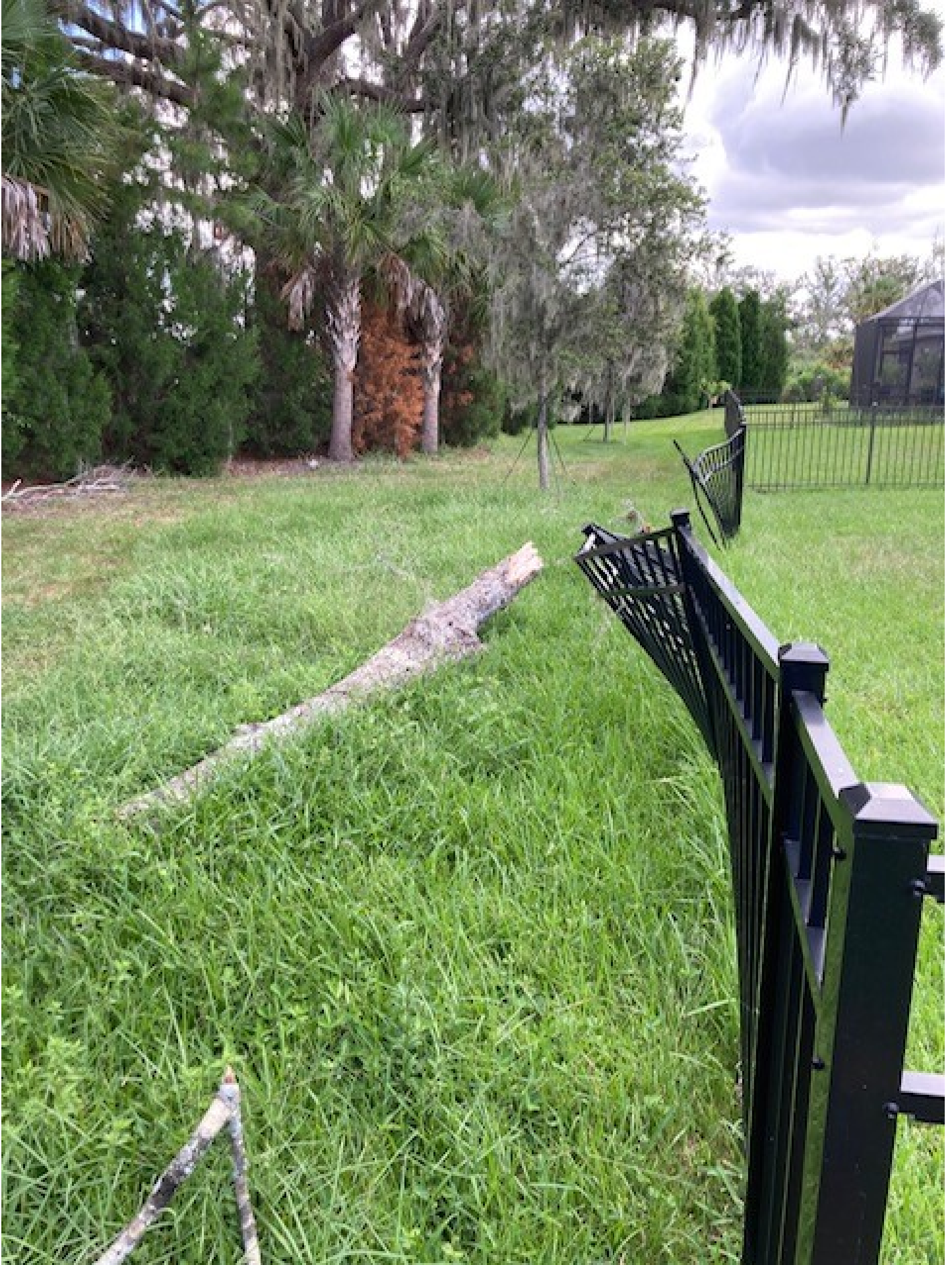
Large Fracture and Fence damage from Dead Oak behind 4840 Deep Creek
