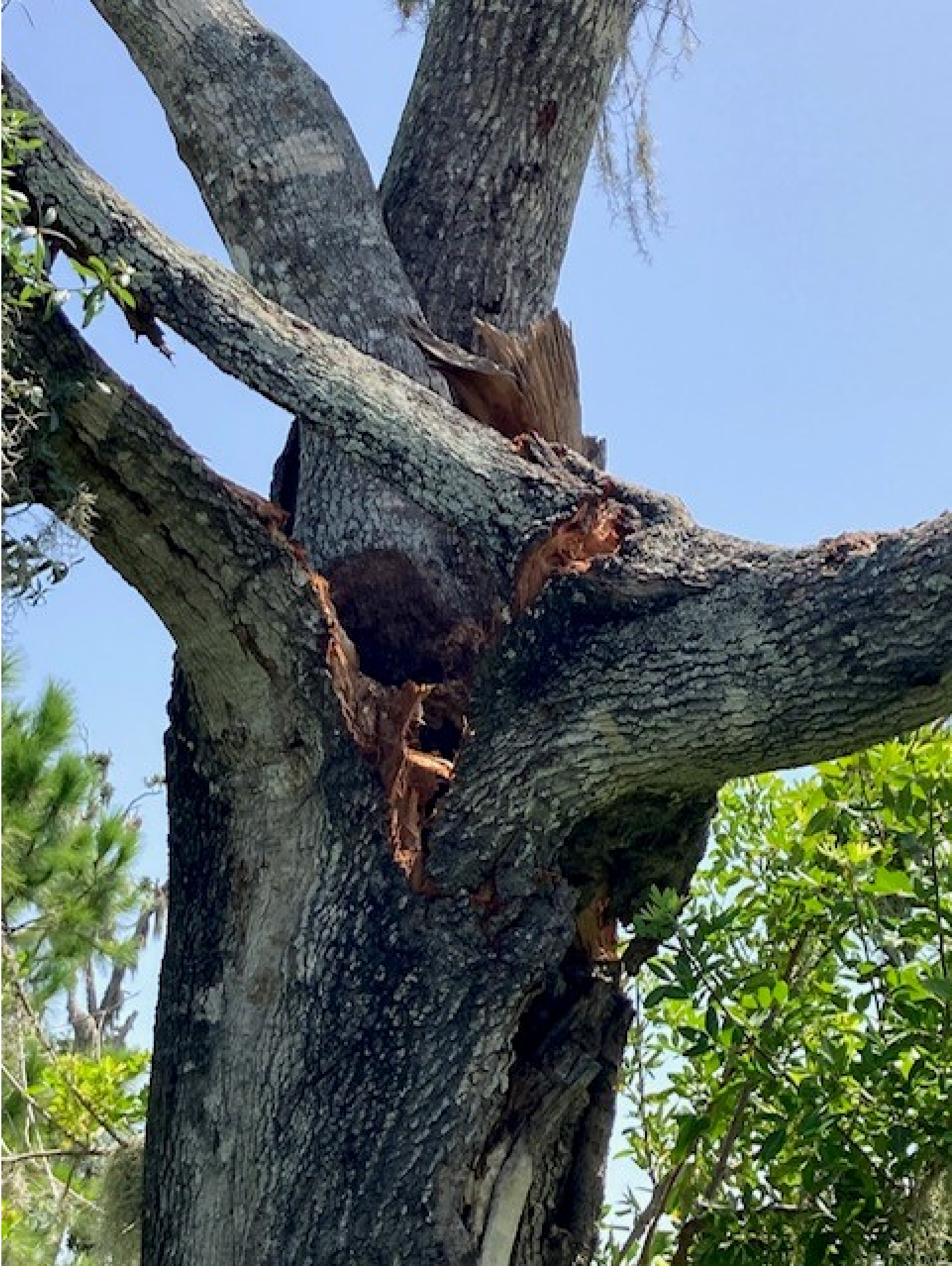
Damaged Branch Attachments of Large Lateral hanging over roof line of 3620 Woodmont Drive
